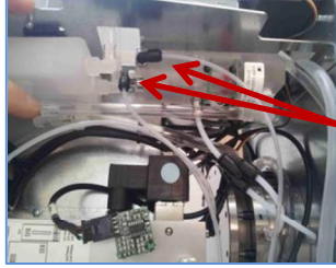
Disconnect pipes on quick connections
